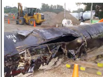
Pipeline which burst in Kalamazoo MI. Spill went undetected for 17 hours. Found by a local farmer.
